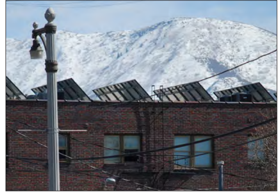
Building utility locations can have unanticipated consequences.
