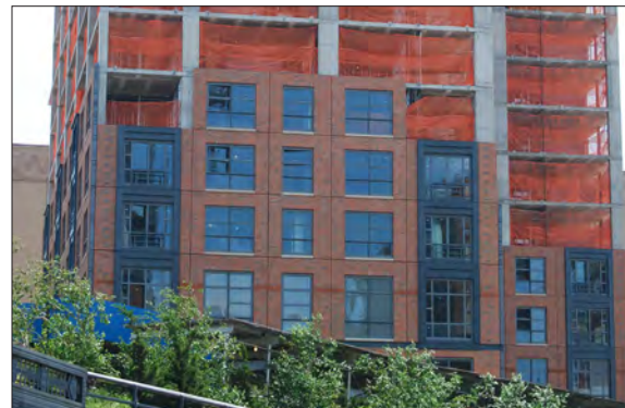
Contrasting dark vertical window bays frame a subtly vertical fenestration pattern in this brick facade.
