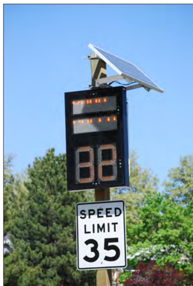
Small scale solar panels and their adaptability.
